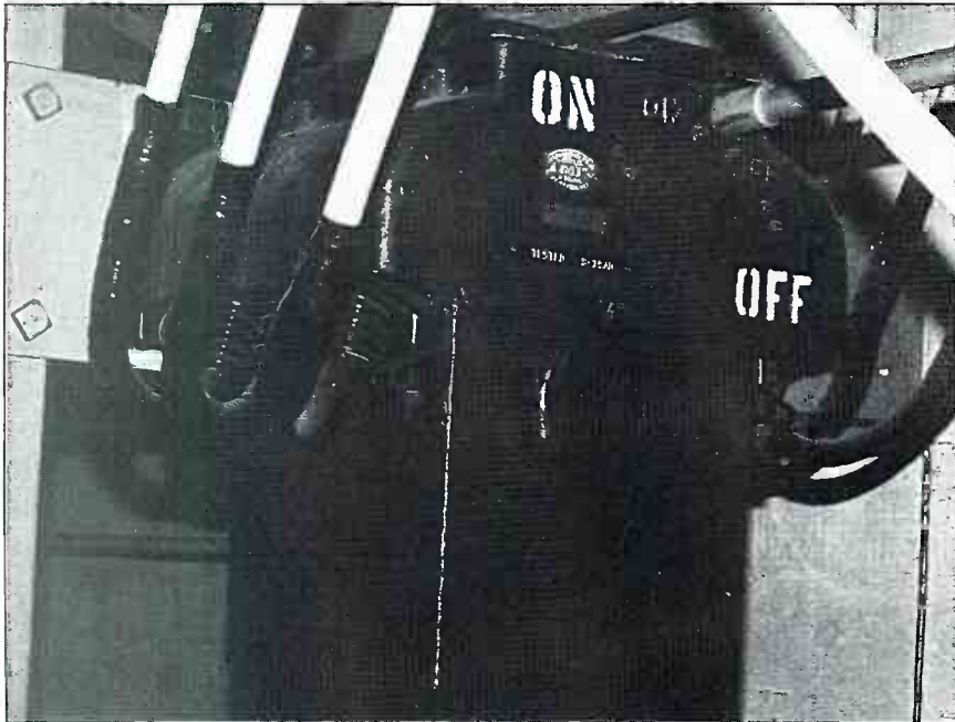
This ac switch was found in the basement of a transmitter building. Note the oil-fill plug on the front panel.
