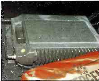
Note the wood base under the transmitter. All trunk-mounted equipment should be secured to a wood or metal base for maximum stability and safety.
