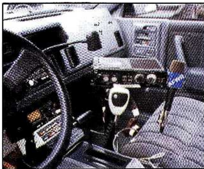
A mobile news vehicle becomes the reporter's office. Closely study the location of the equipment from the standpoint of convenience as well as safety.
