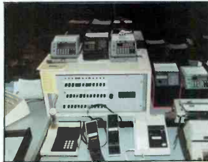
A total of seven receivers, six of which are shown here, places severe demands on any monitoring antenna system. The keys to this installation were careful design and custom amplifiers and filters.
