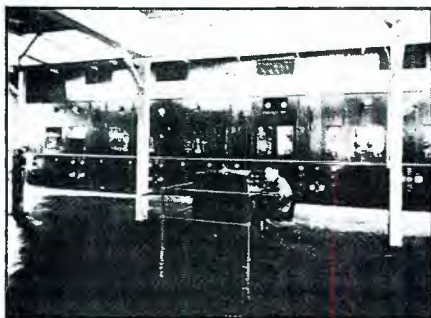
Another view of the WLW transmitter and control console as it appeared in 1934. Full-time operation of the monster 500kW system began on May 2, 1934.
