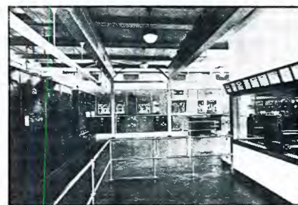
The WLW 500kW transmitter building as viewed from the front entrance. The 50kW exciter can be seen on the left, with the 500kW amplifier-modulator in the background. The audio control room is situated at the right. Circa 1934.
