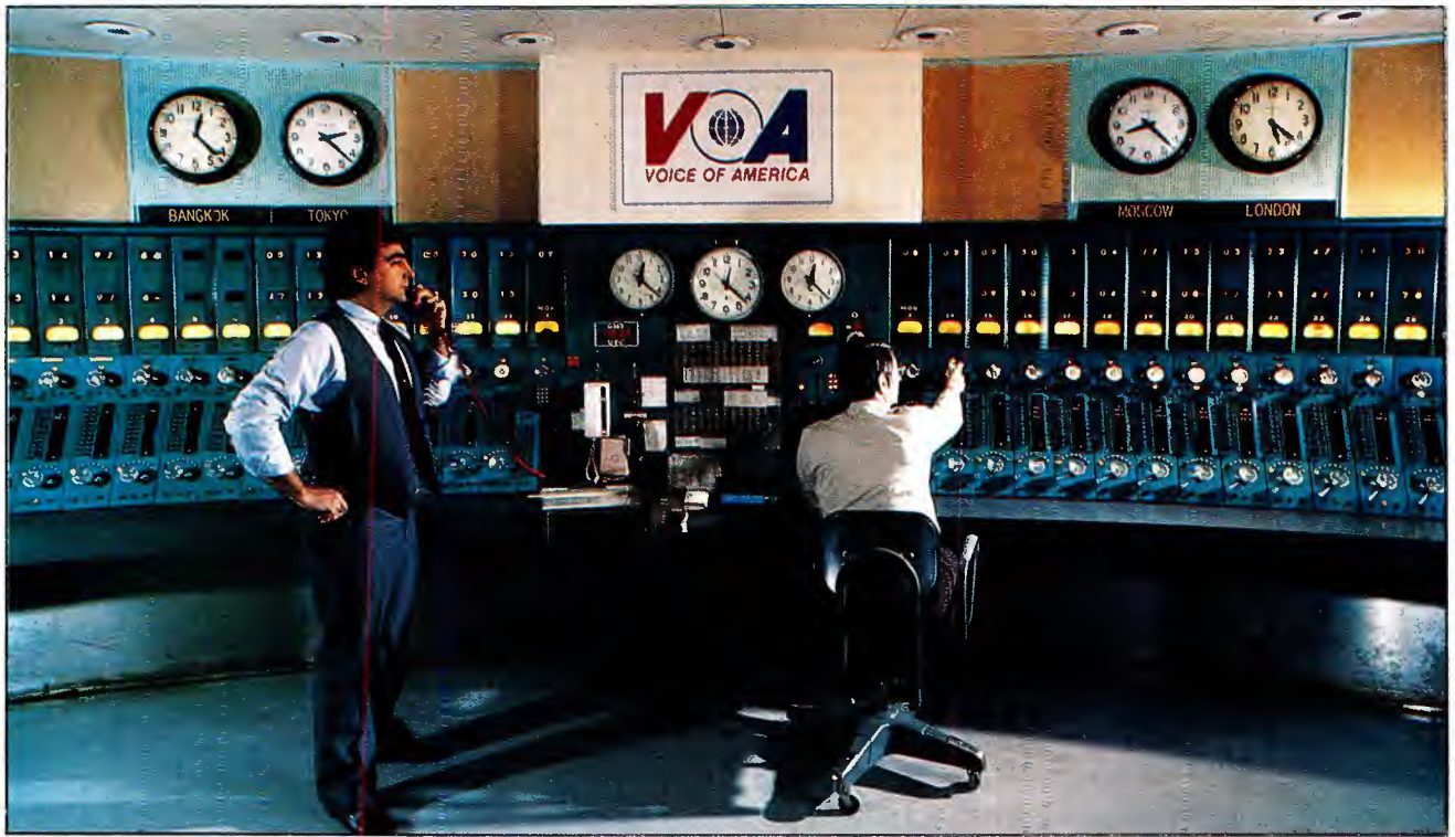
The old Voice of America master control room. Built in the early 1950s, the facility was used until recently to transmit programming in a wide variety of languages to the far-flung VOA system. The equipment shown was designed by Gates Radio to distribute 26 different programs simultaneously from 100 different sources. (Courtesy of VOA.)
