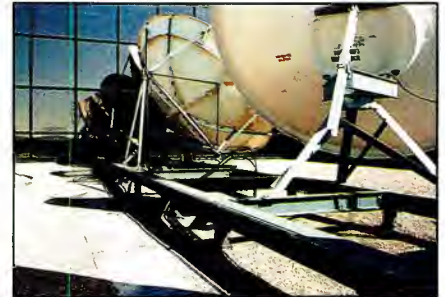
Using a roof-mounted grid allows broadcasters flexibility to update and change outdoor equipment without having to risk damaging the roof membrane.
