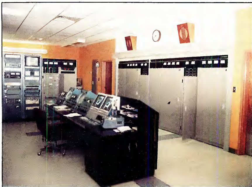
A 120kW Klystrone transmitter installed at WCLP-TV Channel 18 in Chatsworth, GA. (Courtesy of Comark.)
