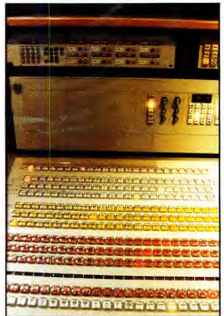
Identical switchers in control room A and B have a router mounted above that can call up any of the 128 sources in house and assign them to eight positions on the switcher. (See eight LED readouts at upper left of photo.)
