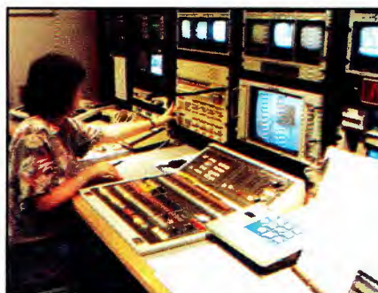
WFTV master control has a router panel with keypad where the operator can call up any of the 128 sources in the house and assign any eight to the small switcher. LED readouts in black windows in the center of the switcher indicate sources assigned.
