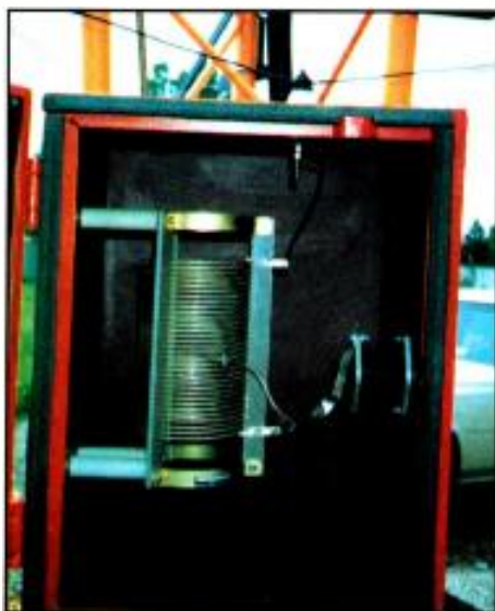
Detuning box containing inductor (left) and capacitor, with base of new tower directly behind. Note detuning skirt wires around tower, terminating at feedthrough insulator on top of box.
