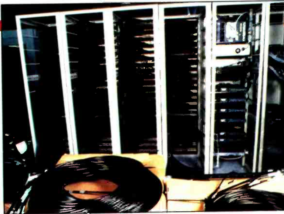
A 200x200 wideband digital routing switcher being installed at Madison Square Garden in New York. Beyond the operational advantages of such a routing system, its physical space requirements are typically less than an equivalent patchbay/DA system would require. (Photo courtesy of BTS.)
