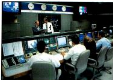
The switching center of a national video fiber-optic distribution system. (Courtesy of Vyvx.)
