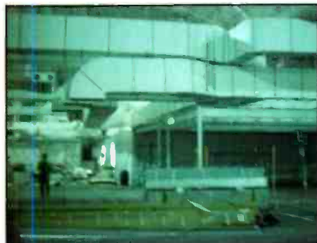
The NBC Olympics Center at the IBC during the early phases of construction. Note the overhead HVAC ducts.
