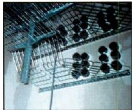
Cable tray assemblies used in the CBS facility. Note the through-wall ports.
