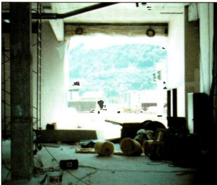
A portion of the CBS broadcast facility at the IBC under construction. The door visible in the photograph is where the two OB trucks entered.
