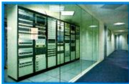
Adding an RDS encoder to the studio racks will allow a station to generate additional revenue. This revenue-enhancing technology is closer than you think. (Photo courtesy of KSAN/KNEW.)
