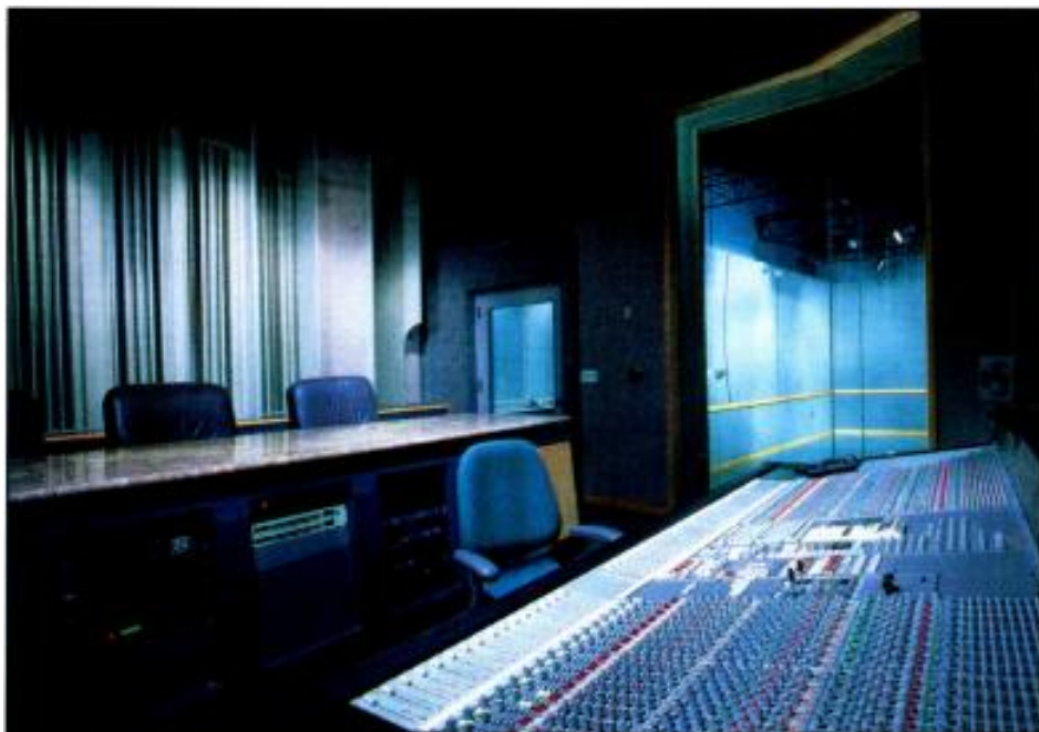
Here a sound-rated door is required to maintain balance with the rest of the facility's sound-isolation performance.
