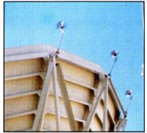
Although a satellite dish is not likely to be struck because of its rounded shape, it may still be vulnerable due to secondary effects of the ground charge rushing to a nearby strike. The dissipation array helps bleed off the accumulated ground charge.
