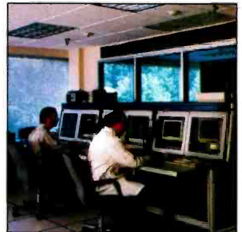
TV Answer's main control room in Reston, VA.
