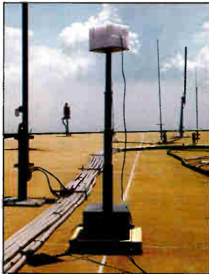
Shown in the 6-foot elevated position, the robot assembly had to make three RF measurements. Signals were interconnected via fiber-optic cable to the spectrum analyzer.
