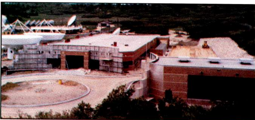
The master uplink and program-origination facility for DirecTV , under construction in Castle Rock, CO.
