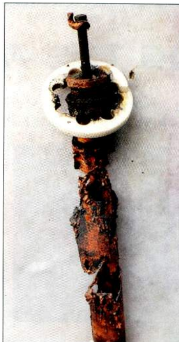
Photo A. Failed inner conductor after removal from WHAS-TV transmission line.
