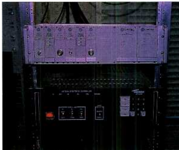
This rack at a station's remote downlink contains fiber-optic terminal equipment (above) and satellite antenna controller (below). (Courtesy of WBBM-TV, Chicago.)
