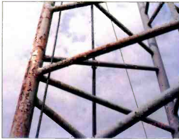
Removing rust to bare metal on a broadcast tower requires an application of a zinc-rich primer. (Photo courtesy of Broadcast Communications, New Glarus, WI.)
