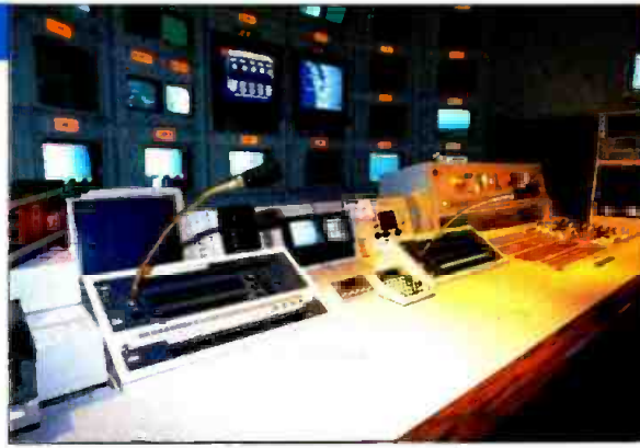
The main production control room at KING-TV, Seattle, with newly installed intercom panels in the foreground.
