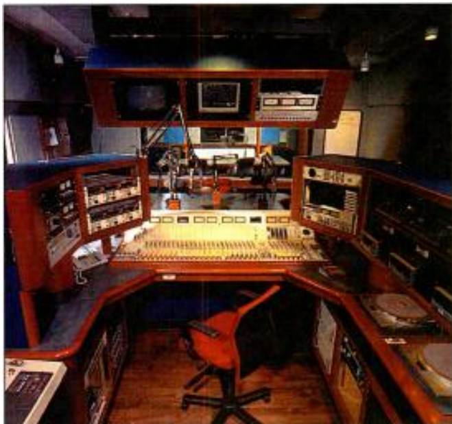
Pacific Recorders and Engineering AMX-34 in the new KABC/KLOS facility, Los Angeles.
