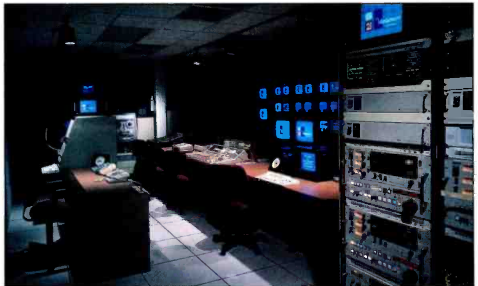
The control room at Montgomery Video Productions helps support a full-service production facility for the Montgomery Community Television cable system. The production capability of many cable systems now approaches that of smaller-market TV broadcasters.
