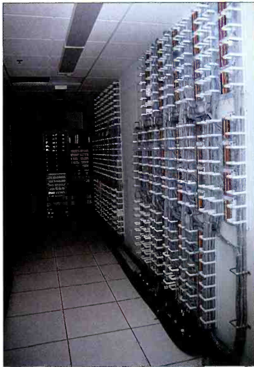
Racks are interconnected with 26-pair cable to wiring blocks mounted on the wall behind each technical area. Computer flooring makes wiring changes a snap.
