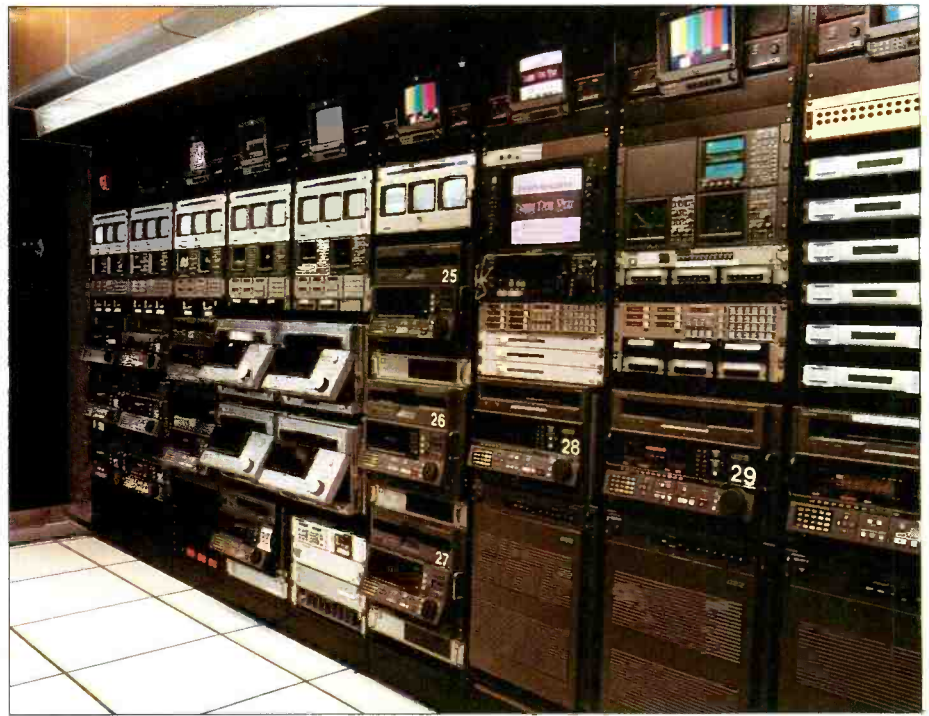
Machine Room A features (left to right) D-2, Ampex DCT and D-1 machines and Imovision encoders for the D-1 decks (at extreme right).
