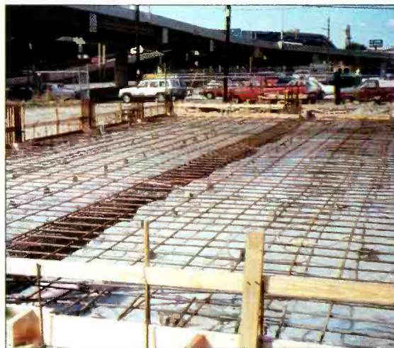
Another shot of the concrete work during construction. Note the expressway on-ramp in the background, a key issue during the site selection. (Photo courtesy of Rees Associates, Inc.)
