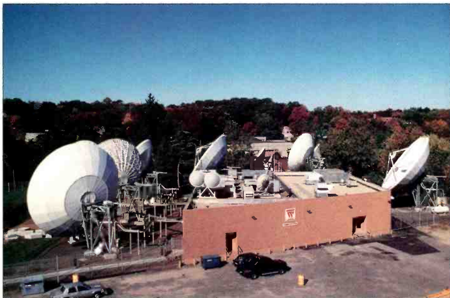
The recently expanded GWNS Glenbrook Earth Station in Stamford, CT.
