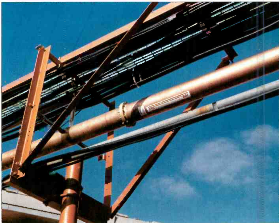
Both rigid coaxial line and semiflexible coaxial cable are included in this transmission line installation at WGTV (Channel 29), Traverse City, MI.
