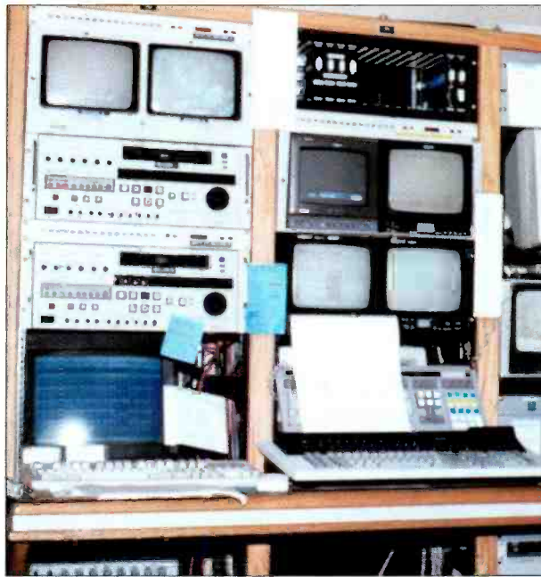
BayTV control room section showing S-VHS record/playback decks and PC-based controllers.
