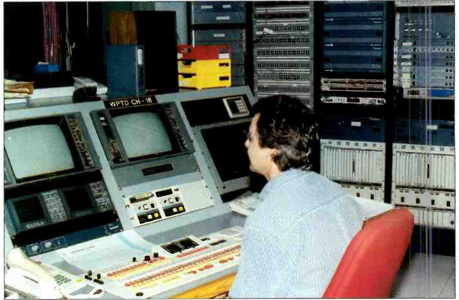
One of the master control stations used at GDPT. The routers and automation units are in the racks in the background.
