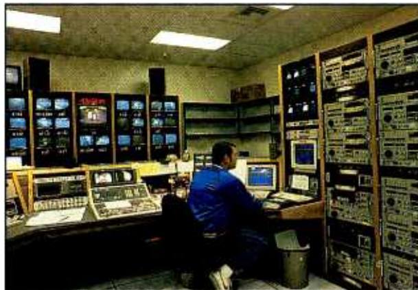
As stations transition from analog to digital, equipment must be chosen carefully to minimize budgeting considerations while ensuring that existing equipment is not rendered obsolete prematurely. (Photo courtesy of Hewlett-Packard.)
