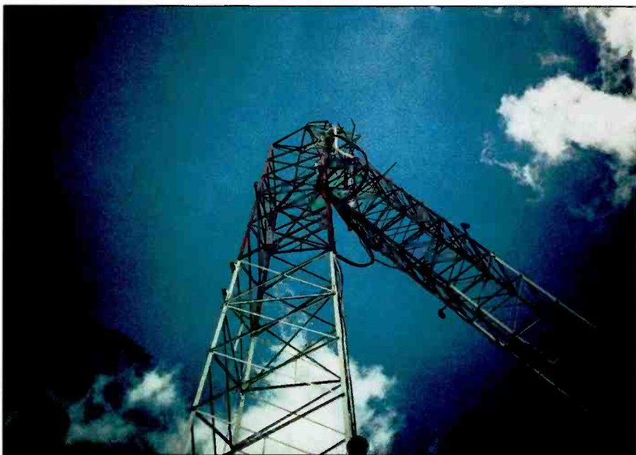
Originally an AM tower, the structure was converted to a paging/2-way tower. All of the new antennas were located at the top of the tower. The tower was not designed for the increased windload and eventual collapse of the tower occurred.
