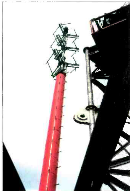
The Channel 3/Channel 21 antenna was assembled and raised into position on the northeast corner of the tower's star mount. (Photo courtesy of Ken Dixon.)
