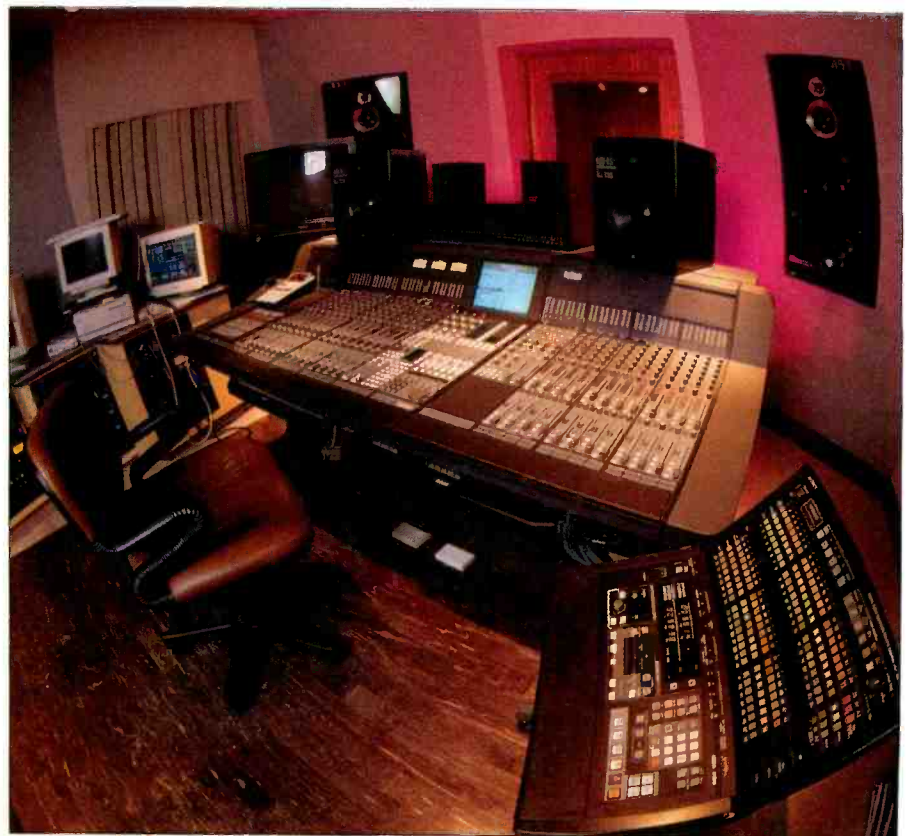
This recently completed post room at Sony Music Studios in New York is based around a 56-fader Euphonix CS2000P mixing system.
