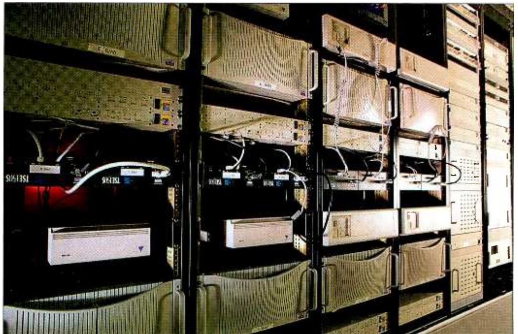
Moving to a server-based environment does not mean you can get rid of all those racks. Considerable rack-mount hardware may be needed, based on your facility's requirements. (Photos courtesy of Avid.)
