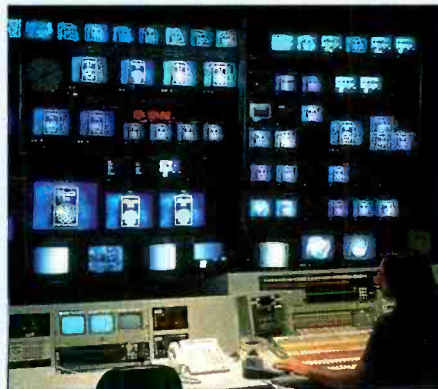
NBC's two main control rooms featured video walls consisting of 124 Panasonic monitors. All of the 171 plus hours of Olympic programming was handled by these two rooms.
