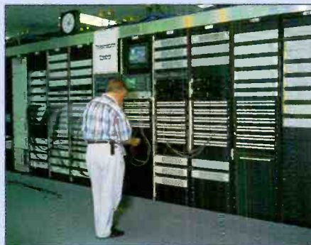
Routing all the signals to the multiple satellite and fiber links was handled in this section of the BOC transmission center.
