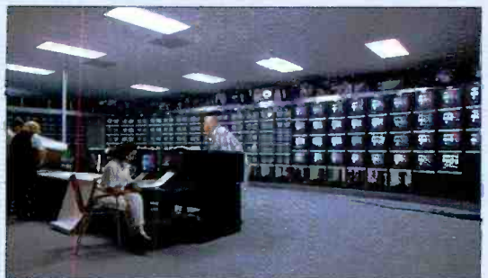
The video feeds were monitored on the video wall in the AOB distribution center.
