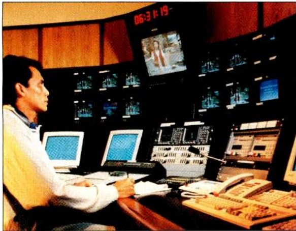
One of the master control rooms at ABC Singapore, a state-of-the-art multichannel facility.
