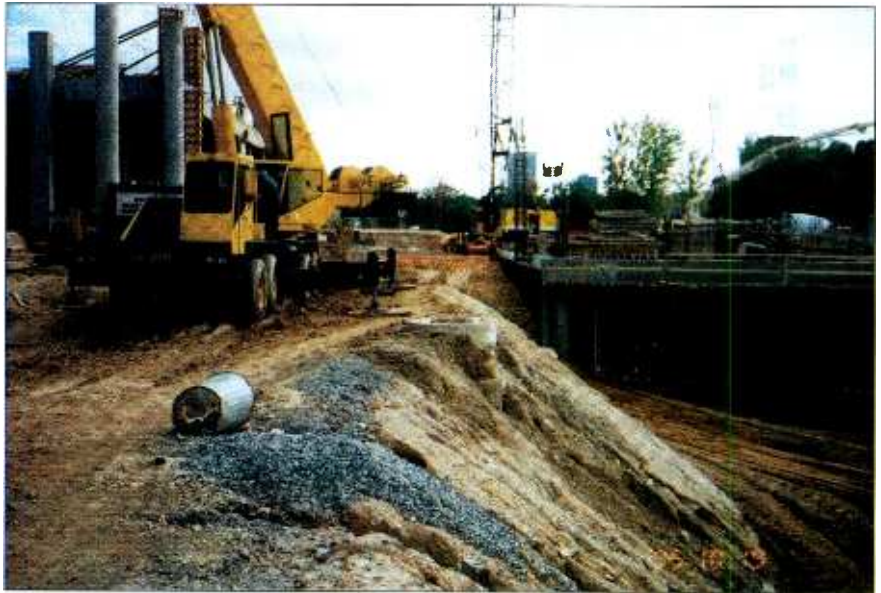
Nearly 70,000 square feet of the building was constructed beneath the parking deck.
