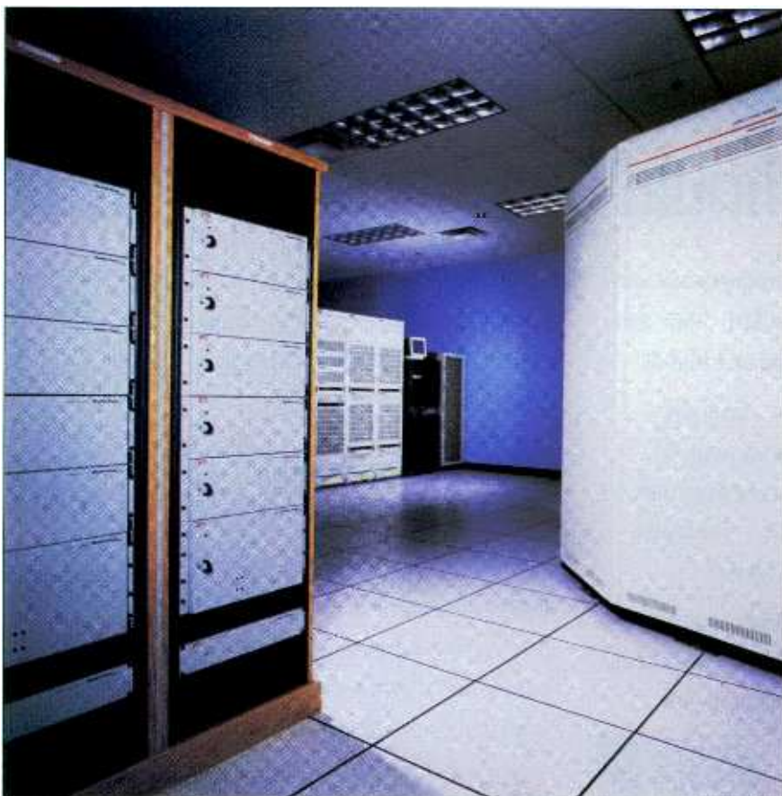
In the Speer facility, a seven-channel and an eight-channel Media Pool store content required for real-time playback.
