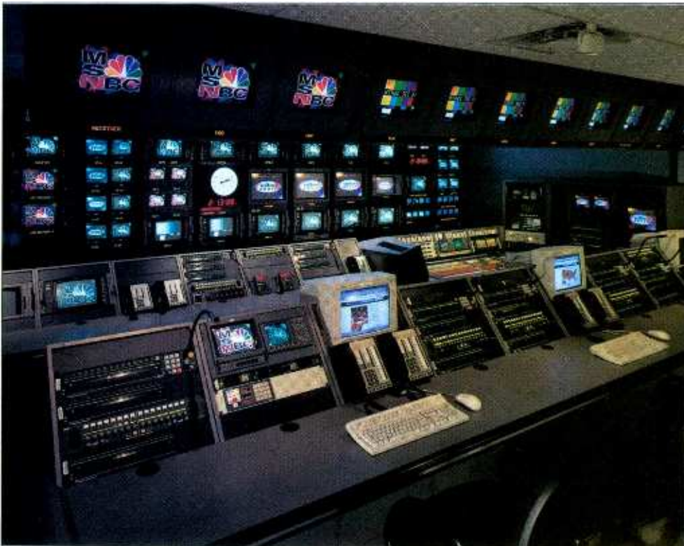
One of the two production control rooms currently installed. Provisions exist for a third control room if needed.
