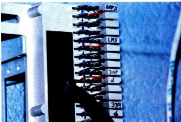
A 10BASE-T network uses RJ-45 cable connectors and punchblocks, which makes installing a UTP network straightforward.
