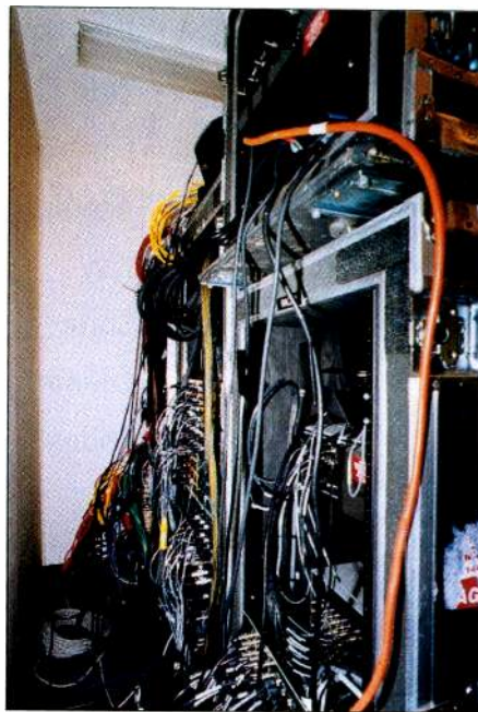
Despite its appearance, wiring for the Sony racks is well marked, and easy to connect.
