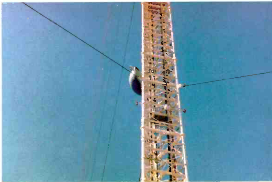
Intermediate tower lights can no longer be installed on the tower. Existing towers are "grandfathered," but new towers must have two fixtures installed so that at least one light is clearly visible without any obstruction from the tower members.
