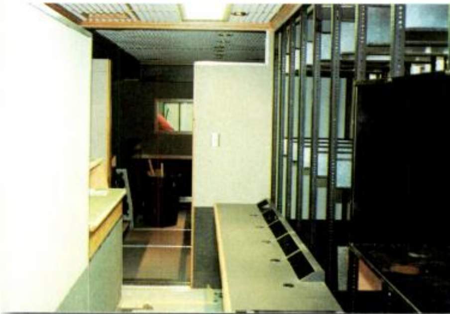
The videotape and control area contain nine racks. The first five racks, shown above, contain five HDW-500 recorders and associated monitors. The next four racks provide video control for up to 16 cameras. Note the large black box on the right. It is used to house one of two HDM-20E1U high-definition monitors.
