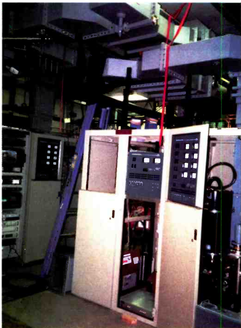
The WKAR transmitter site in Lansing, MI, is home to this transmitter from Advanced Broadcast Systems.
