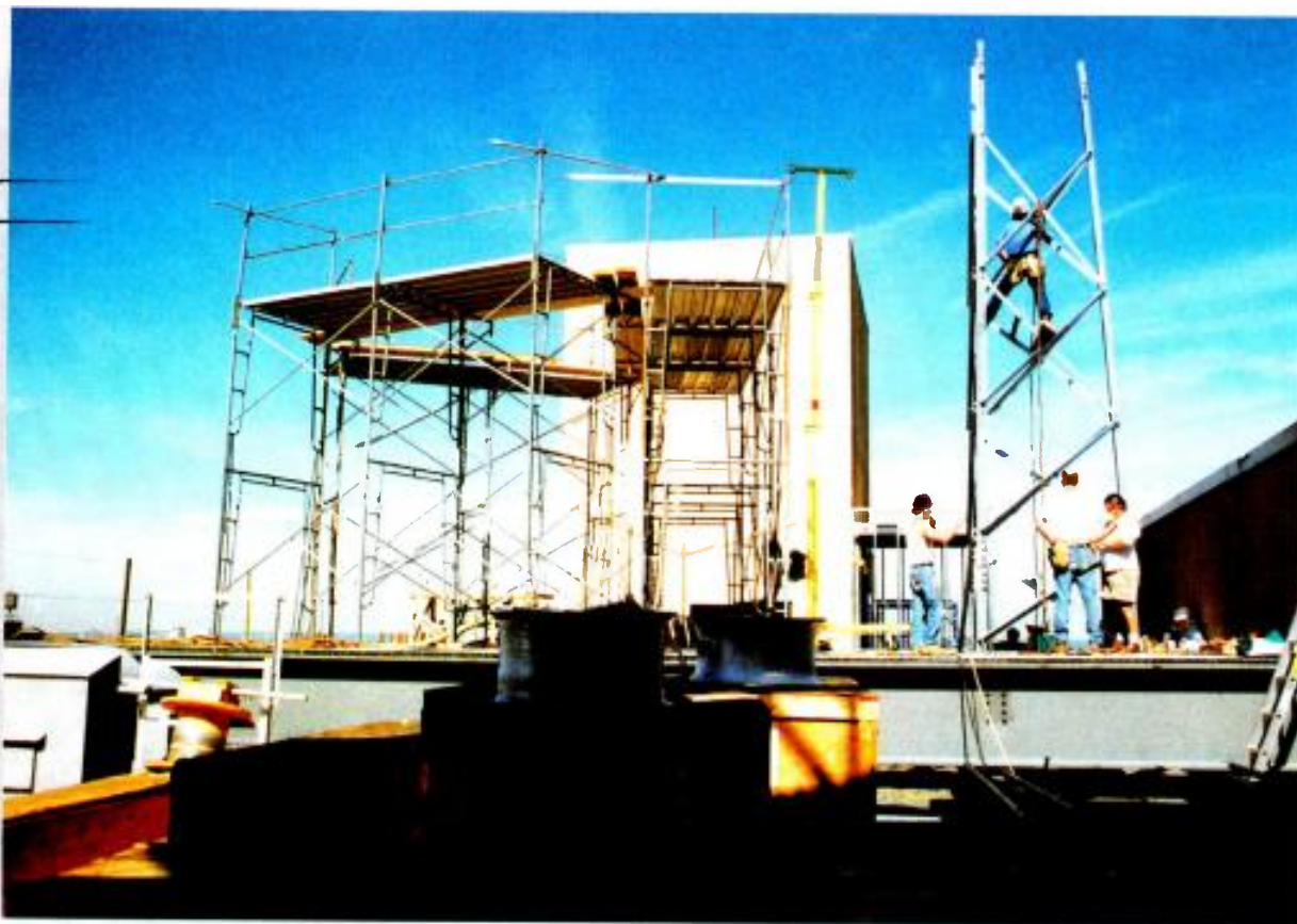
Rooftop RF support for 7.6m steerable and 7.3m fixed receive-only satellite antennas, assorted VSAT and DSS antennas, plus a 60-foot microwave tower.
