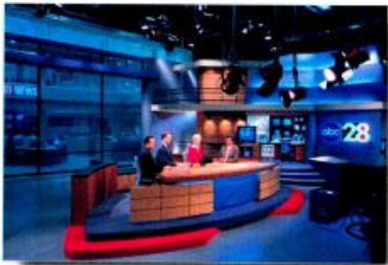
Systems integrators are playing a larger role in new facility design such as this studio located at WFTS-TV and built by Professional Communications Systems.
