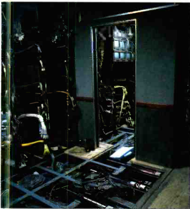
Much of the initial integration work involves getting the correct cables to the proper locations. Note the heavy-gauge welded cross members in the floor. Bolted construction will not stand up to the rigors of road work. (Photo credit: Concept: Benson and Rice)
