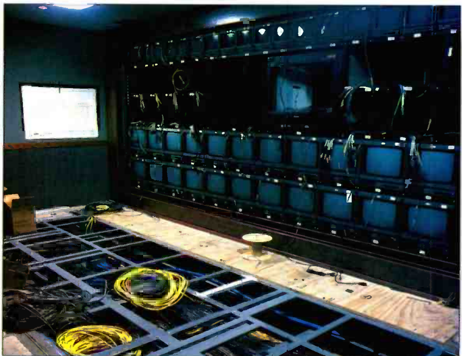
Miles of wiring lie behind the racks and floors. Shown is the production control room during construction. The completed room is shown on page 92. (Photo credit: Concept: Benson and Rice)
