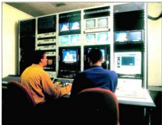
One of the two NOAT control rooms. Louth Automation and the Grass Valley model 101 master control switcher are shown.
