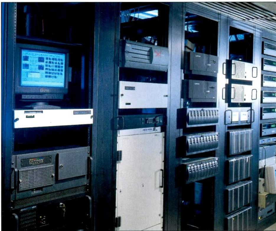
Rack room showing a news ASC server, a Grass Valley Group routing switcher, and the station's ASC server.
