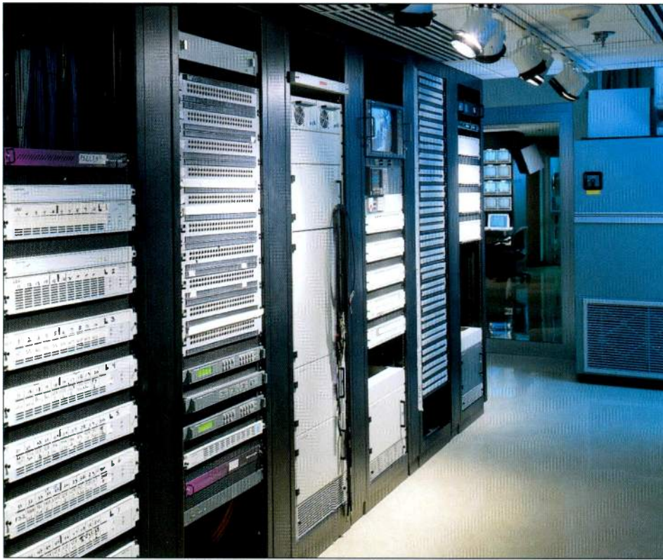
Rack room showing distribution amps, patch panels and a Leibert computer room air conditioning unit in the background.
