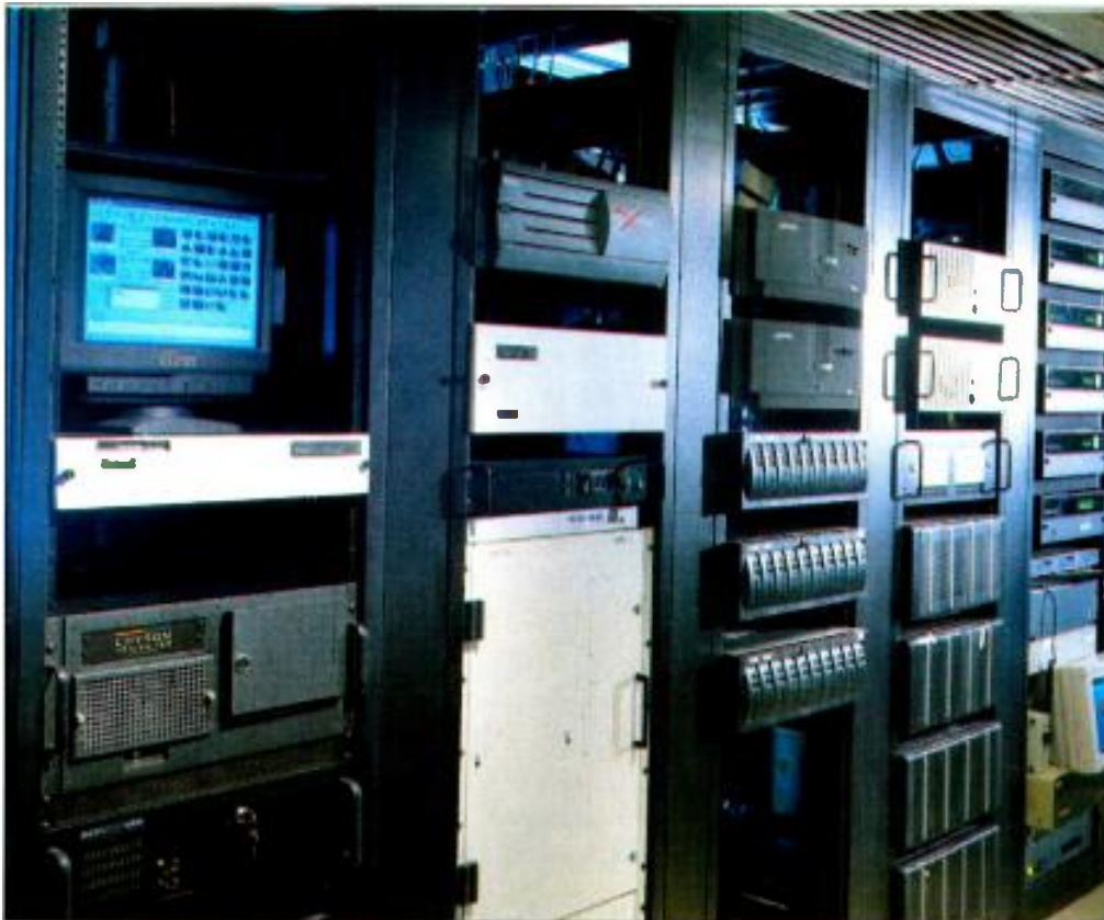
Rack room showing a news ASC server, a Grass Valley Group routing switcher, and the station's ASC server.
