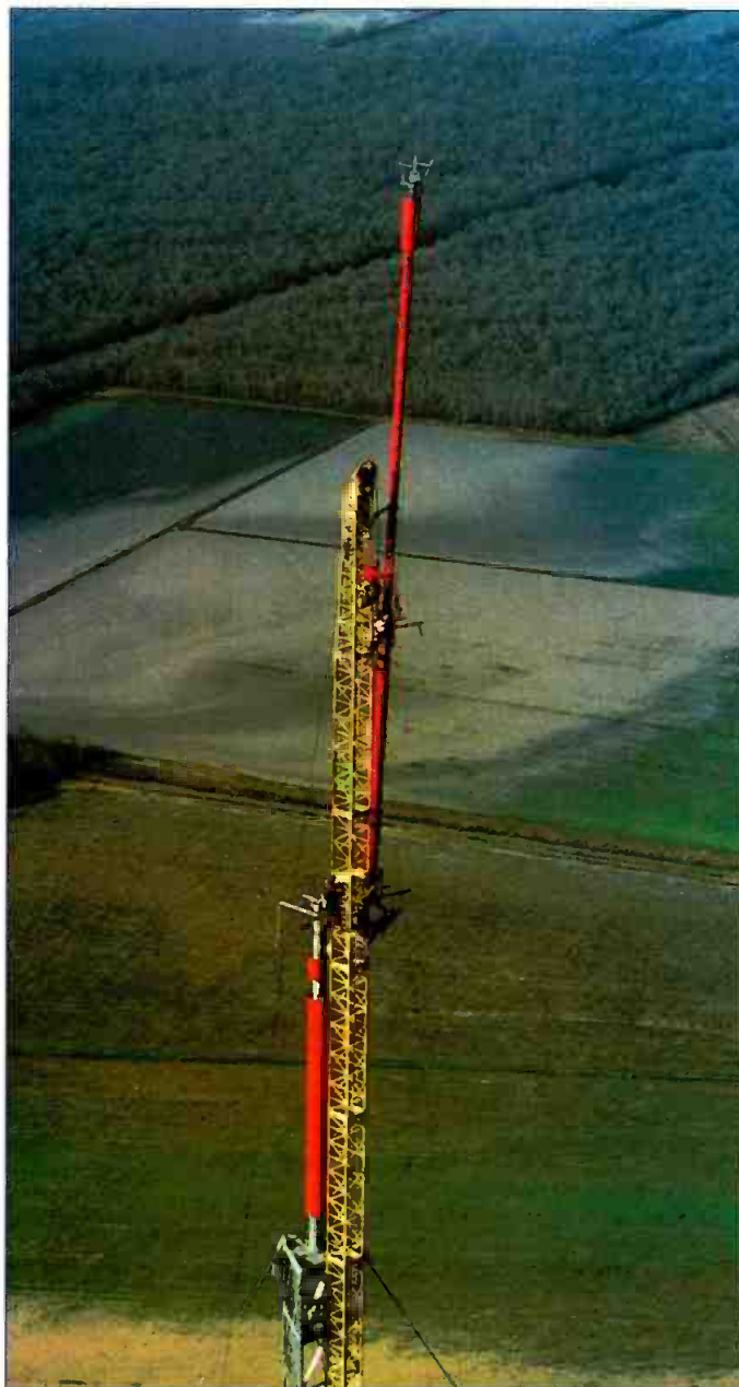
Photo of the installation of a 17-ton Dielectric traveling wave antenna on the nearly 2000-foot KNOE-TV tower near Monroe, LA. Photo courtesy LeBlanc Broadcast.
