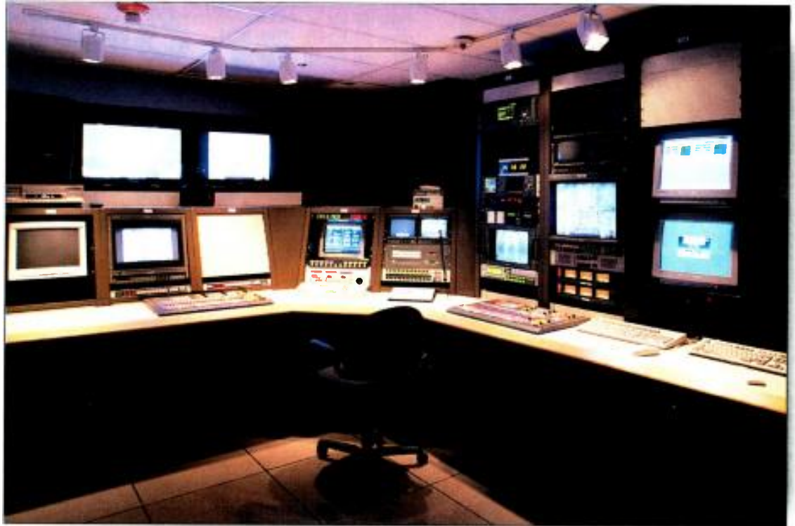
DTV facilities must handle several layers of data, including video, audio, control and metadata, plus legacy analog signals. KHOU, Houston, routes both standard and high-definition signals through its dual master control rooms. Photo courtesy of Tektronix.
