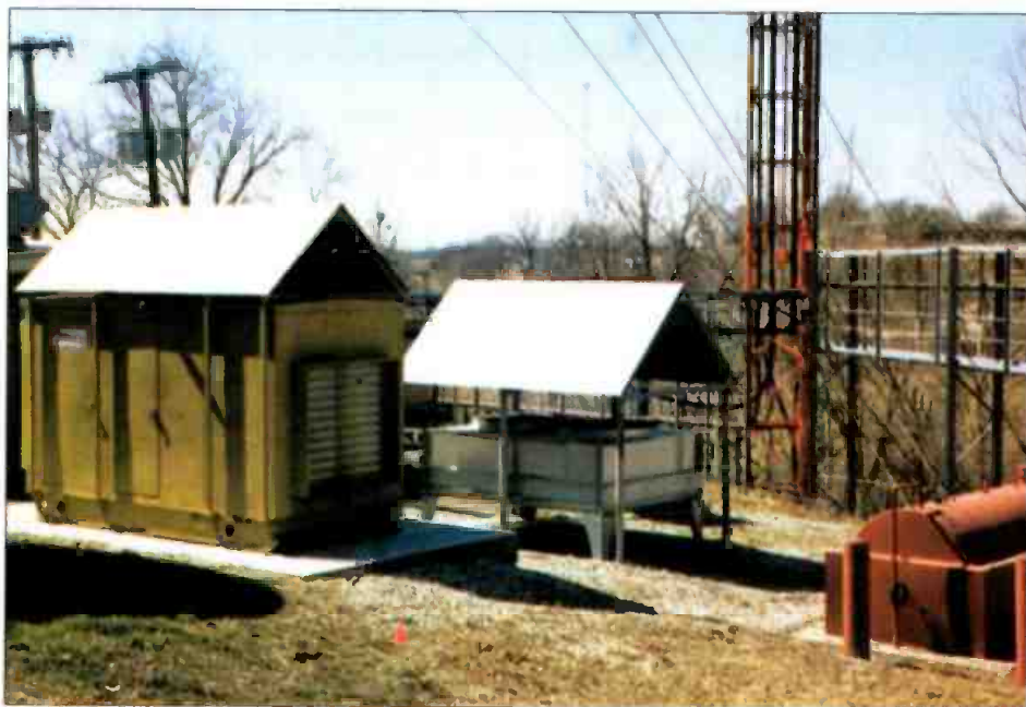
In addition to the tower, there are numerous other items such as outdoor heat exchangers, generators and the generator's fuel supply that all need to be readied for the cold weather ahead.
