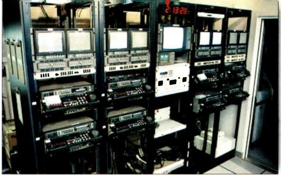
Included in WLWT's rack room are Panasonic DVCPRO decks for recording and playback tasks.
