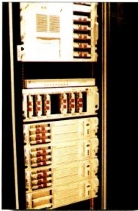
One of the many computer systems currently used to serve Web info, along with its associated storage. The entire system is built with redundancy and fault tolerance as a priority.
