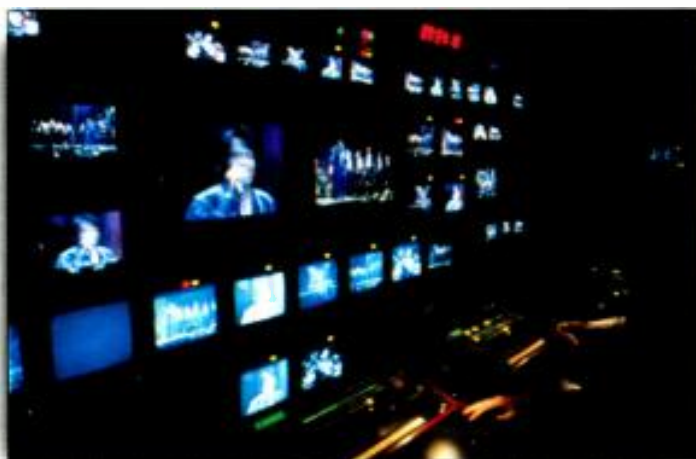
The HD video control room in the NMT HD-2 production truck, installed by Sony Systems Integration Group. (Photo courtesy of Sony)
