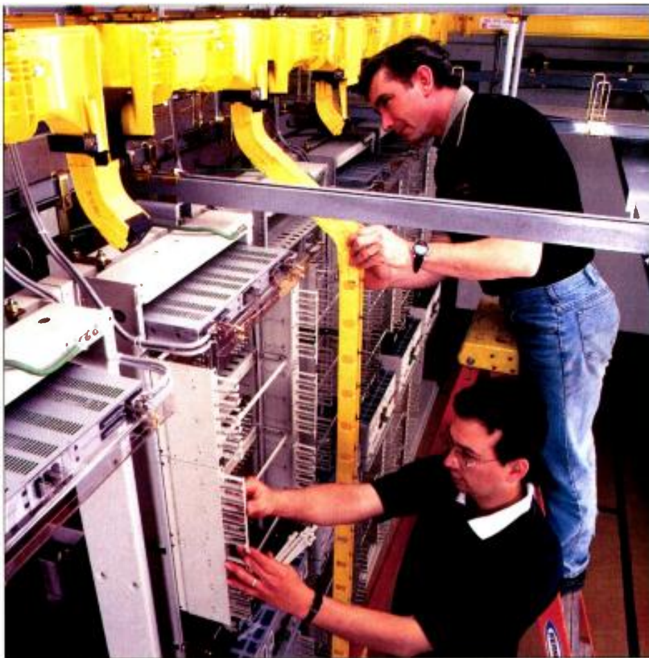
While installing fiber cable, strict adherence to guidelines regarding its flexibility must be observed. Raceways, such as those being installed here, help to organize and protect cable, as well as ensure the integrity of its location and minimum bend radius over time. Photo courtesy ADC Communications.
