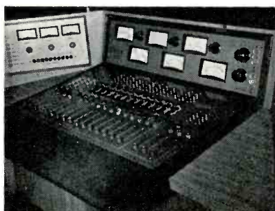
Fig. 5. Horizontal Control Panel with Slide-type Mixing Pots.
