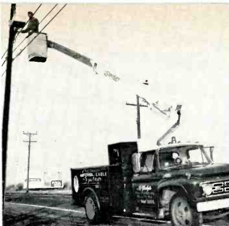
Econovan equipped with Servi-Lift facilitates maintenance of Atlantic's pole-mounted amplifiers.
