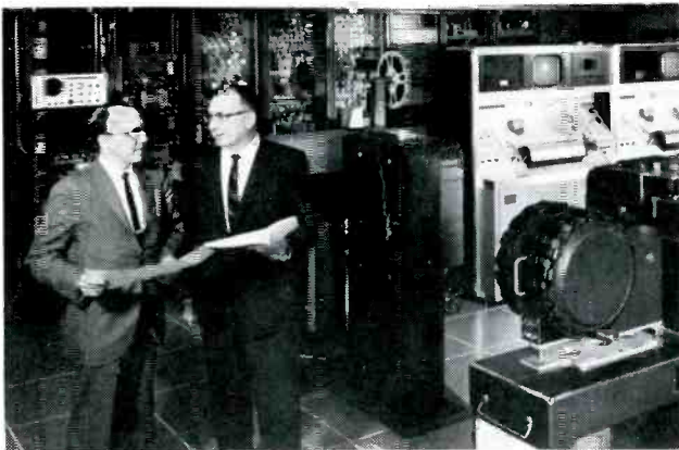
Asst. C.E. Art Vrooman and C.E. Ted Campbell in equipment room at WJAC-TV.
