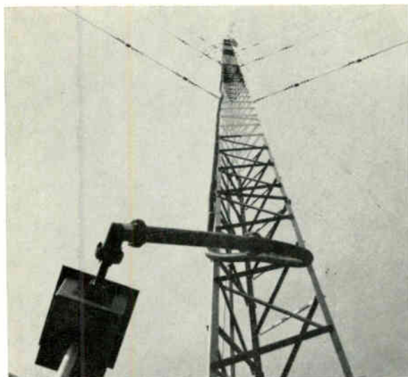
View of 326-ft Collins 37M-11 a-m tower with isolation coupler in foreground. The 11 bays of fm antenna are mounted at the extreme top of the tower.
