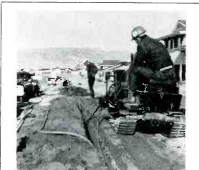
Vumore Video, Inc. is busy building a 412-mile underground system in Colorado Springs, Colorado.
