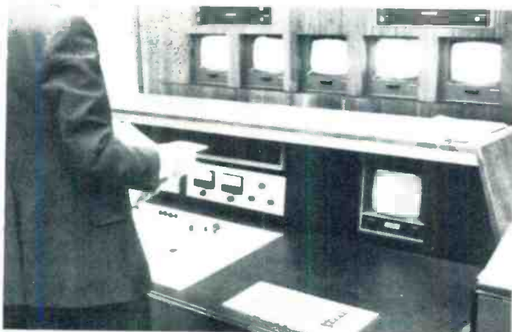
Grass Valley's TV switching automation system.
