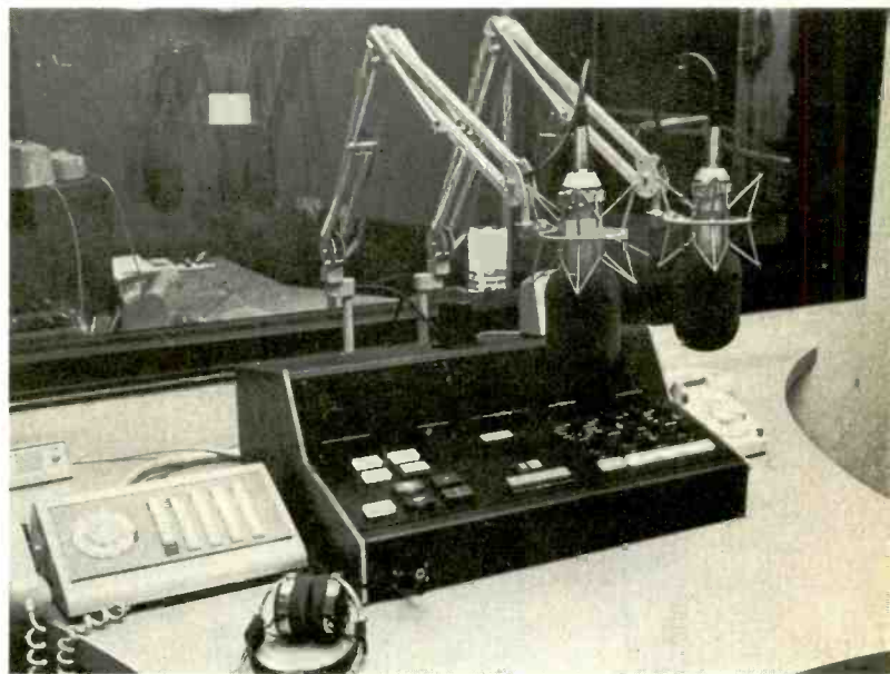
Studio A control room has turret for controlling talk shows.
