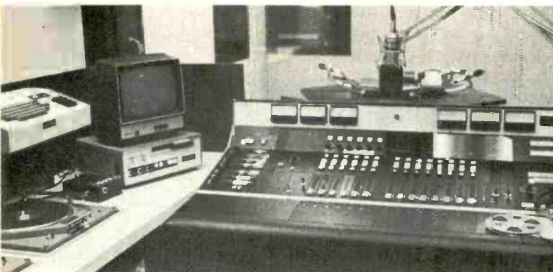
The AM-FM interface board, with the talk studio in background. The console is a completely dual board, for either stereo or mono—two programs can be handled simultaneously.
