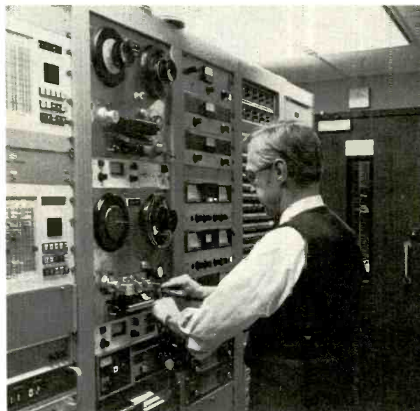
Central equipment rack, with Tom Whalen, technician, changing heads on Ampex 351 tape transport.
