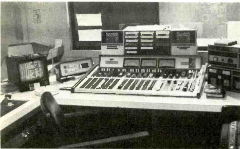
CRT display of upcoming events is located at the master control board.
