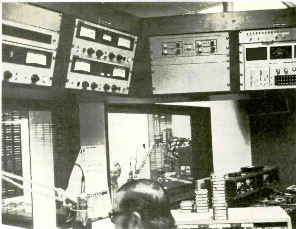
To the left and below right, are two views of the master control at WBEN. Top view shows the adjustable height overhead turret, which holds remote control and monitoring equipment for AM and FM transmitters. Below view shows a corner of the console and the cart machine bank.
