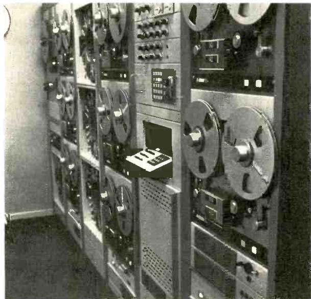
The SMC DP-1 automation system feeds most of the programming to the FM station, but any origination point in the plant can feed either the AM or FM transmitter.
