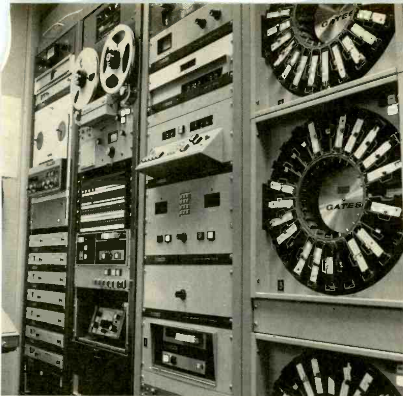
Two racks to right in photo show part of main equipment used for automation at WERE. Harris (Gates) control, memory, and electronic switching equipment are in third rack; three of the seven rotary cart machines are visible in the fourth rack.
