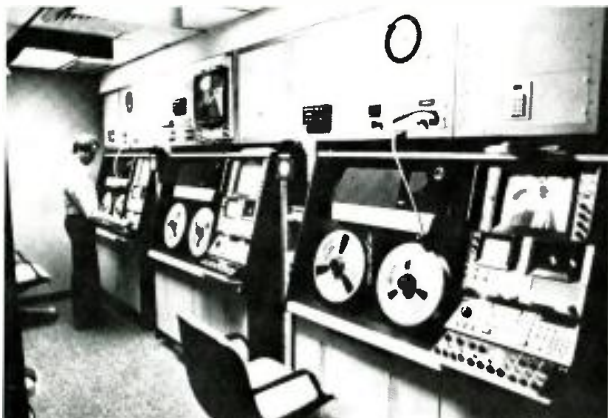
AVR-3s are housed in environmentally controlled room and form the basic VTR capability for ABC's facility.
