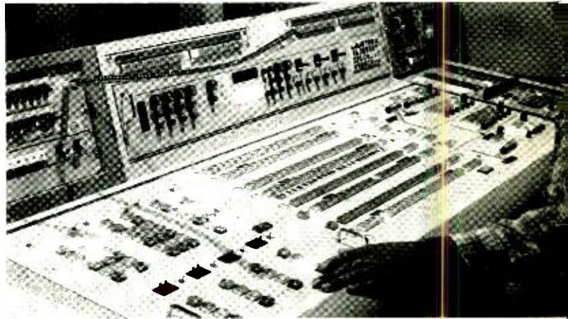
Machine control panel, Grass Valley switcher, and Vital SqueezeZoom in news studio control room at KPIX
